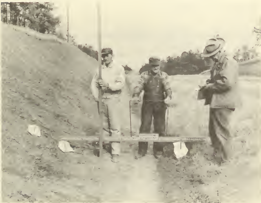
Figure 6.--The specially designed surveying equipment is being used in connection with metal hub stakes for measurement of erosion or sedimentation in the flow channel.
